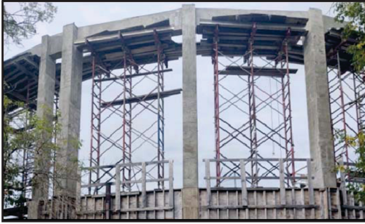
FOUR COLUMNS COMPLETED FROM THE SACRED SPOT AND GOING EAST TO THE LEFT
