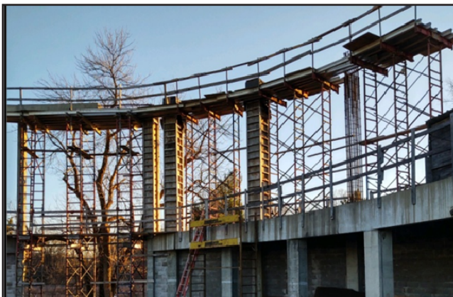
THREE OF THE FOUR COLUMNS WITH THEIR FORMS ATTACHED MAKES FOR A GOOD START
