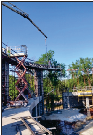
POURING FIRST FOUR COLUMNS AND CONNECTING ROOF-SUPPORT BEAM (Volunteers now work toward accomplishment #4)
