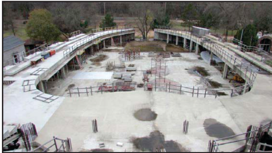
MEZZANINE FLOOR COMPLETED (Volunteers now have accomplished: Lower Floor + Main Floor + Mezzanine )
